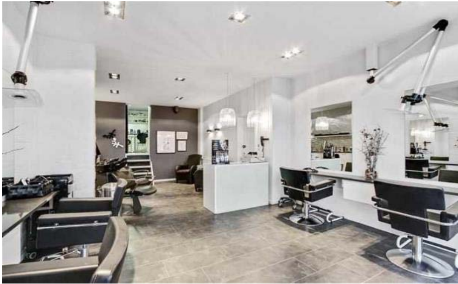
A salon with appropriate local exhaust ventilation
